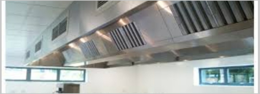
Kitchen Ventilation System
